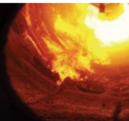
View into the hot end of a rotary cement kiln during production. Raw materials are heated to 1400-1500°C.
